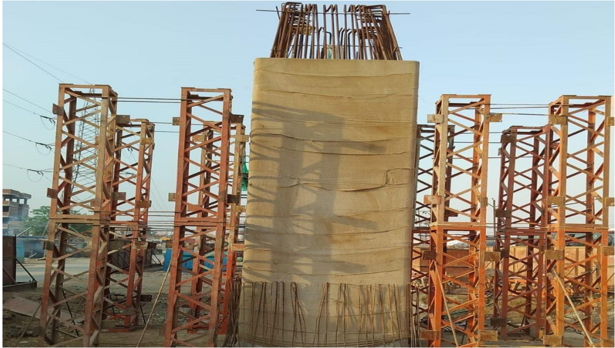
Fig : Preparatory works for Erection of Platform cross arm at Patliputra Bus Terminal Station
