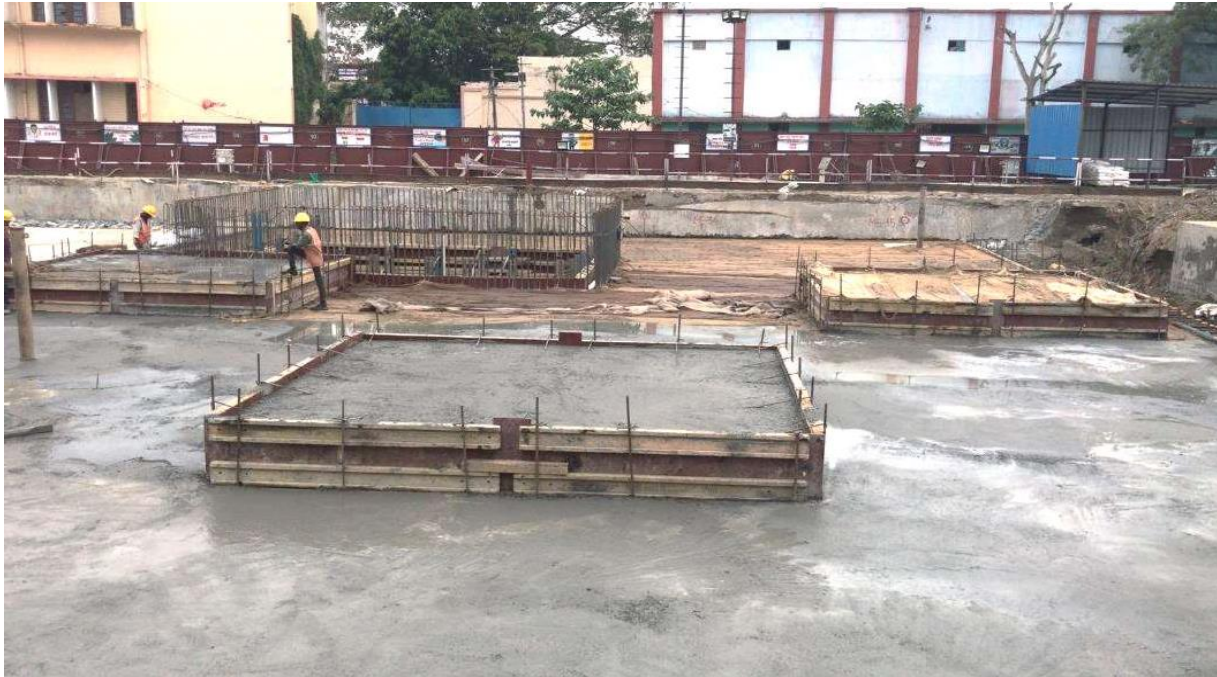
Fig : Roof slab works in progress at Moin Ul Haq stadium Station
