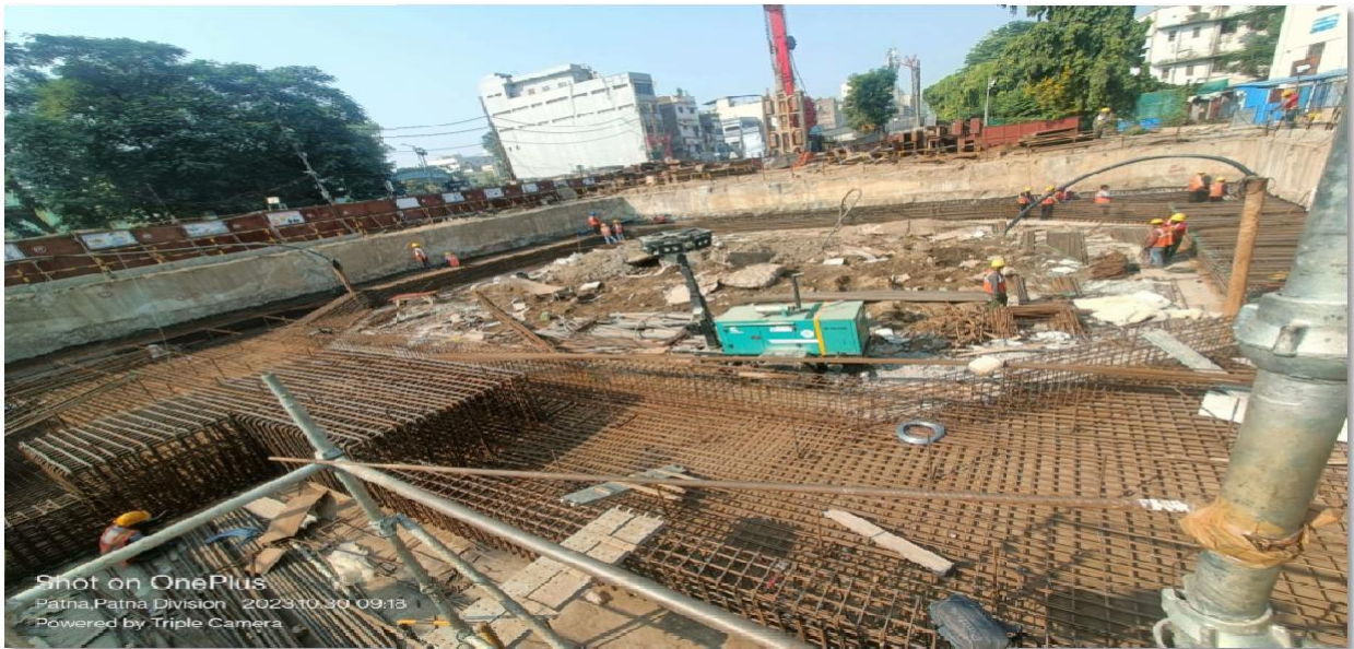
Fig : Launching Shaft Roof slab Reinforcement work in Progress at University Station
