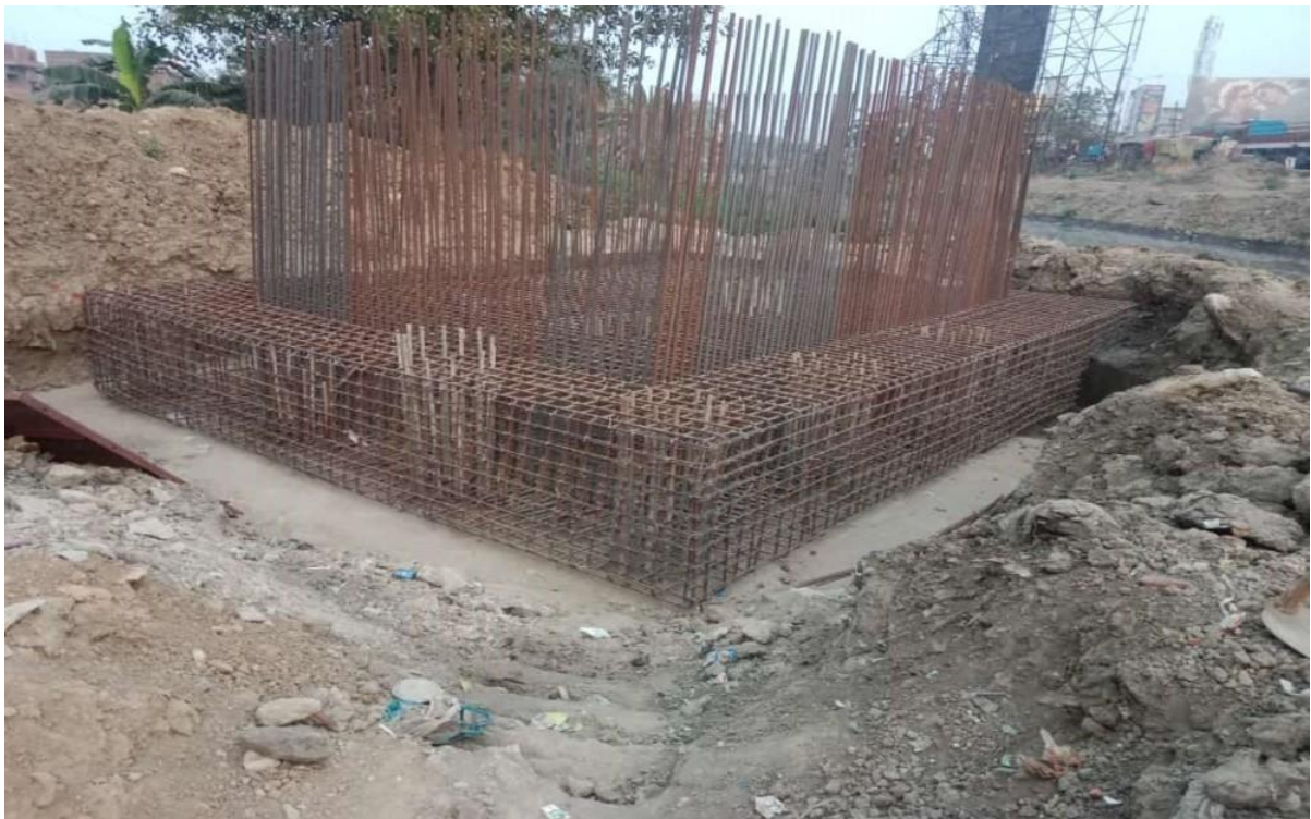
Fig.: Pile Cap work in progress for shifting of existing 132 kV double circuit transmission line of BSPTCL
