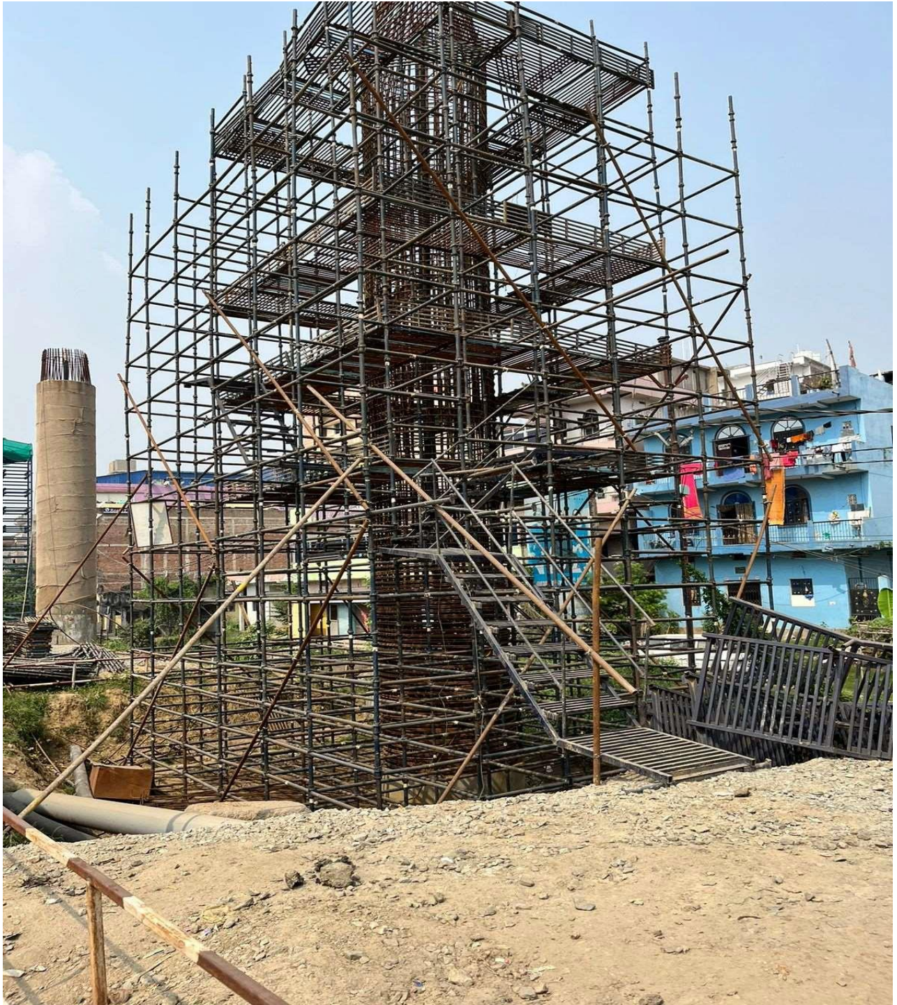
Fig.: Pier reinforcement work in progress between Mithapur to Ramkrishna Nagar Station
