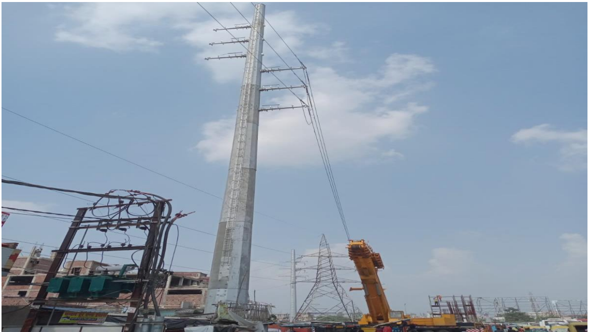
Fig.21: Erection of Monopole and Diversion of electrical utility in progress at project sites of Patna Metro Rail Project
